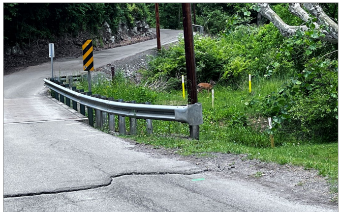
Rotan Street that extends from downtown Fayetteville to the Love Hope Arts center and The 304 restaurant is in need of pedestrian improvements. Photo Credit: Consultant Team/EP&A
